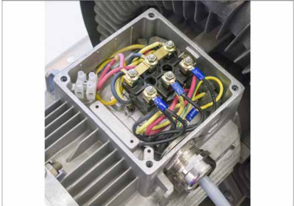
Wiring at the motor connection box
