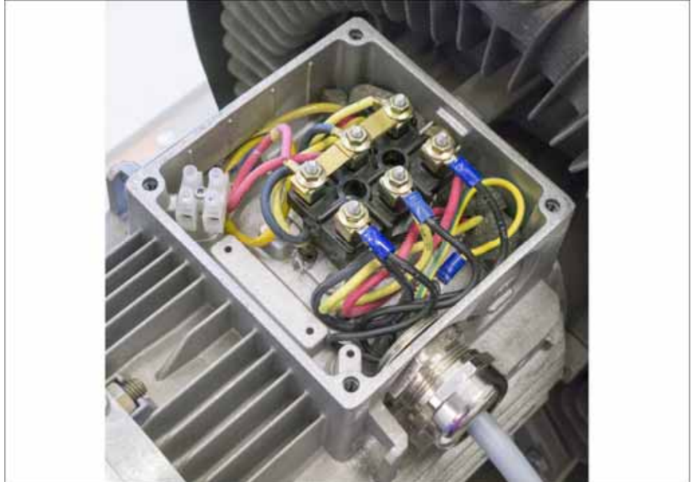
Wiring at the motor connection box
